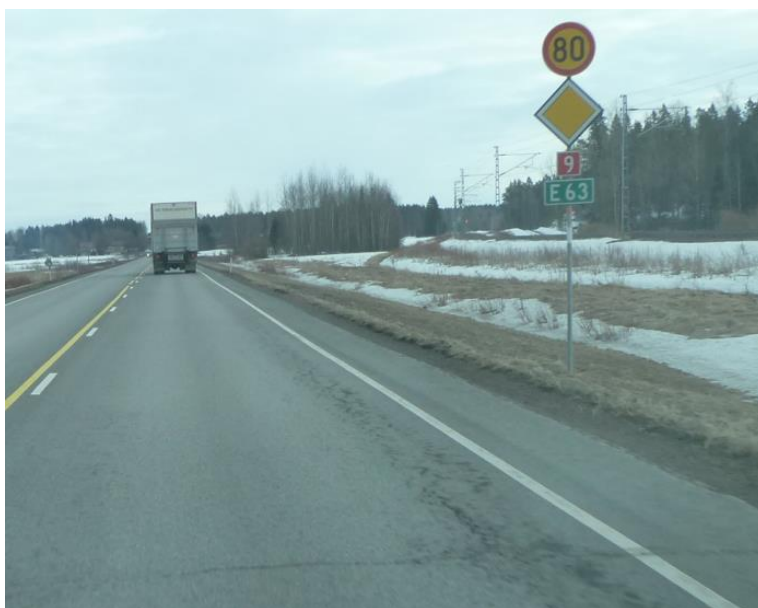
Figure 1: Top down cracking is a typical new pavement damage in Finnish roads after super single tyres have been taken into general use.
