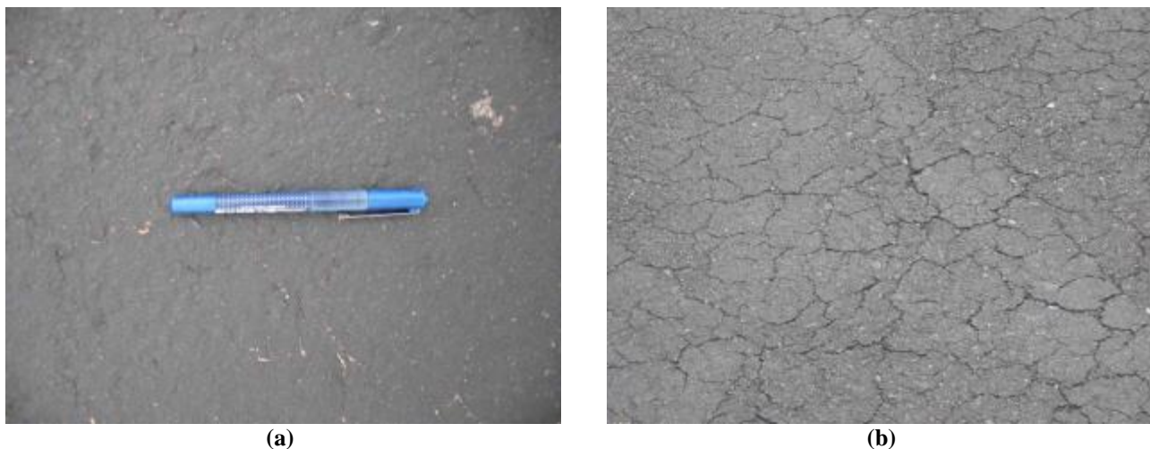
Figure 5: Examples of (a) slippery and (b) cracked fuel resistant membranes
