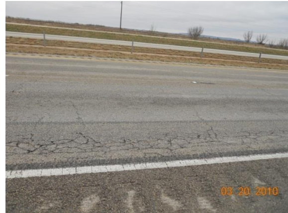
IH 20: PM with porous layer over seal coat due to fatigue cracking (High ADT)
