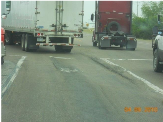
FM 1472: RH with base repair and rigid pavement due to severe rutting (High ADT)
