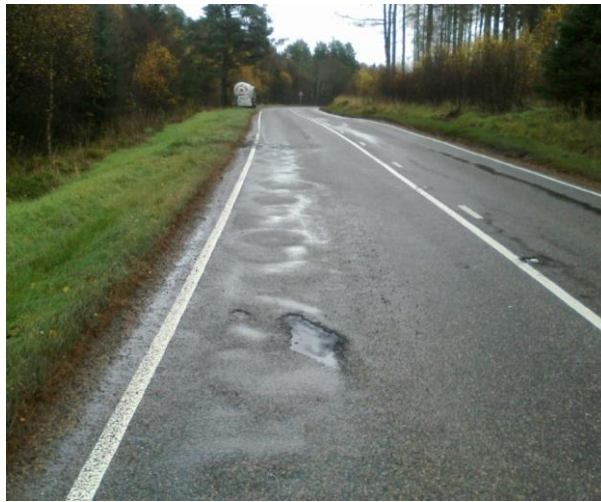
Figure 3: Pothole or substantial road repair?
