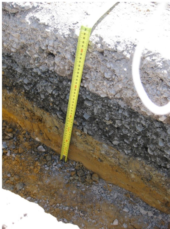
Figure 5: Moisture in subgrade
