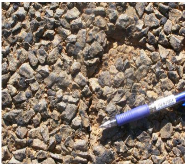
Original cracked pavement
