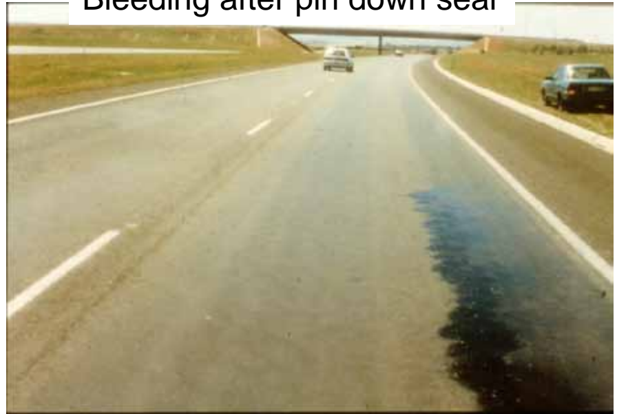
Bleeding after pin down seal
