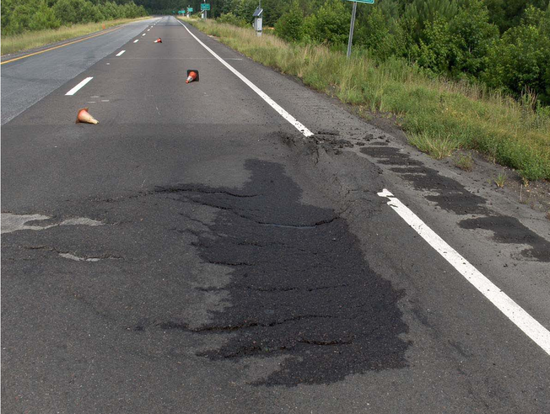
Figure 9: N8 Pavement failure after conventional mill and inlay at 4 million ESALs. [19]
