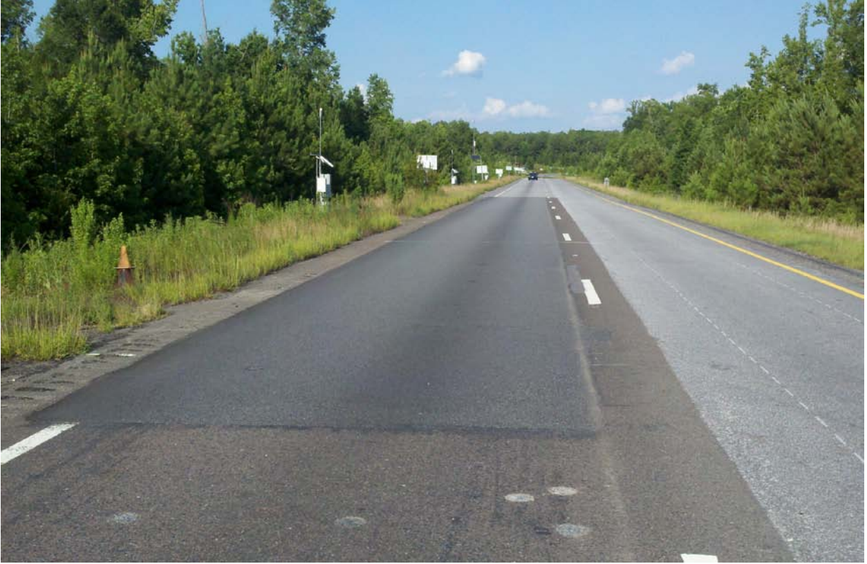
Figure 11: Current state of section N8 with highly modified surface after 4.2 million ESALs.
