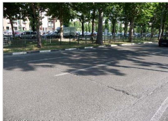
Fig. 11: Unreinforced area in July 2009
