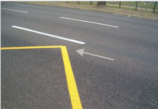
Fig. 9: First signs of cracking in the unreinforced area in May 2006
