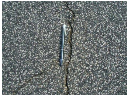
Crack at same width as host - 6mm (No host surface preparation)
