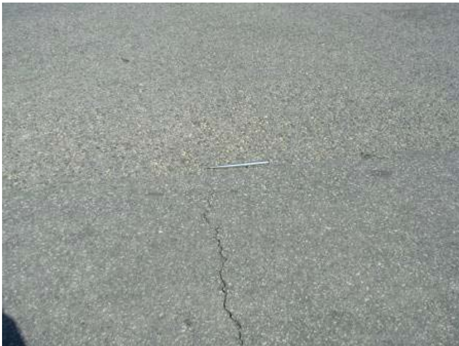
Cracking in Section 1 GG but not in SMA (after 2 years)
