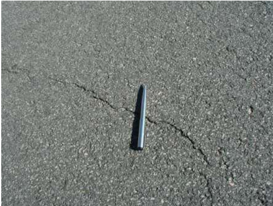
Cracking Section 2, dense graded AC (after 2 years)
