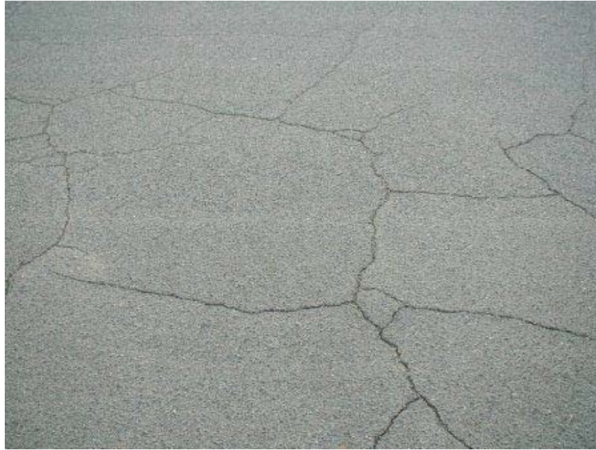
Typical block cracking
