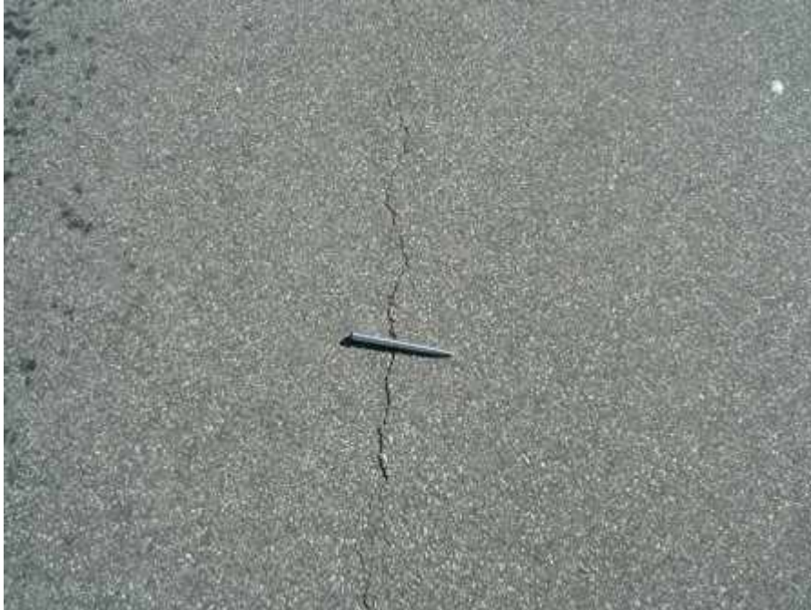
Cracking Section 2, GG AC (after 4 years)
