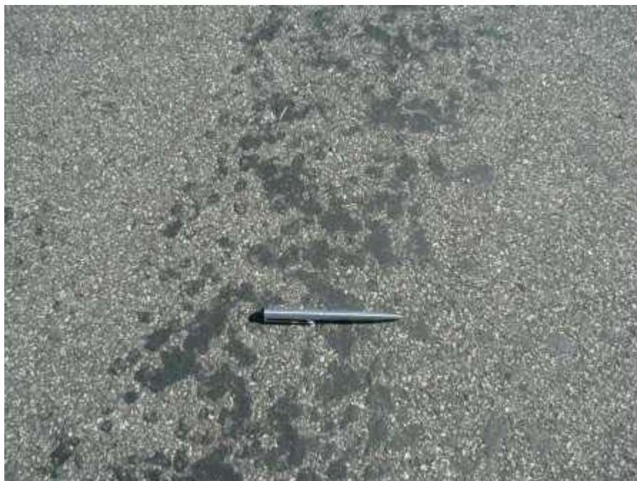
Flushing in Section 2, GG AC (after 2 years)
