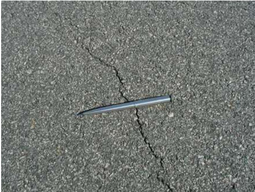
Cracking in section 1, dense-graded AC (after 2 years)
