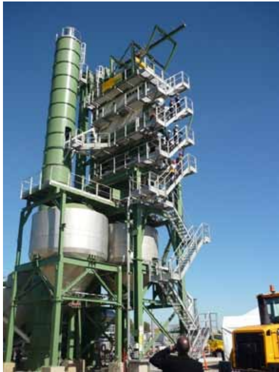
New Boral Asphalt Plant Ballarat Vic
