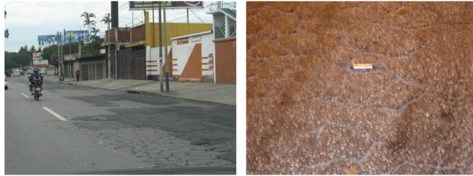
a) Abundant cracking.
