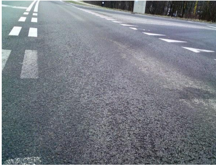
Figure 1: Example of ravelling of a thin surfacing at a junction.
