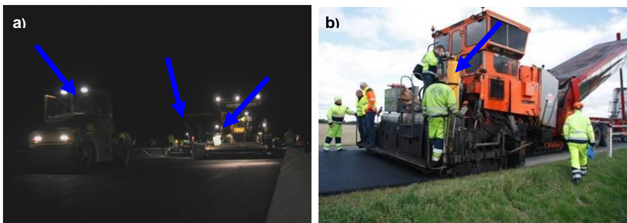
Figure 3 Placement of air emission detectors for the three different positions on the BBTM example (a) and on top of the paver for the SMA example (b).
