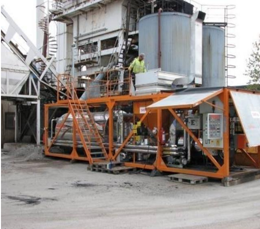
Figure 1: Crumb rubber and rubber blender connected to an Asphalt plant.
