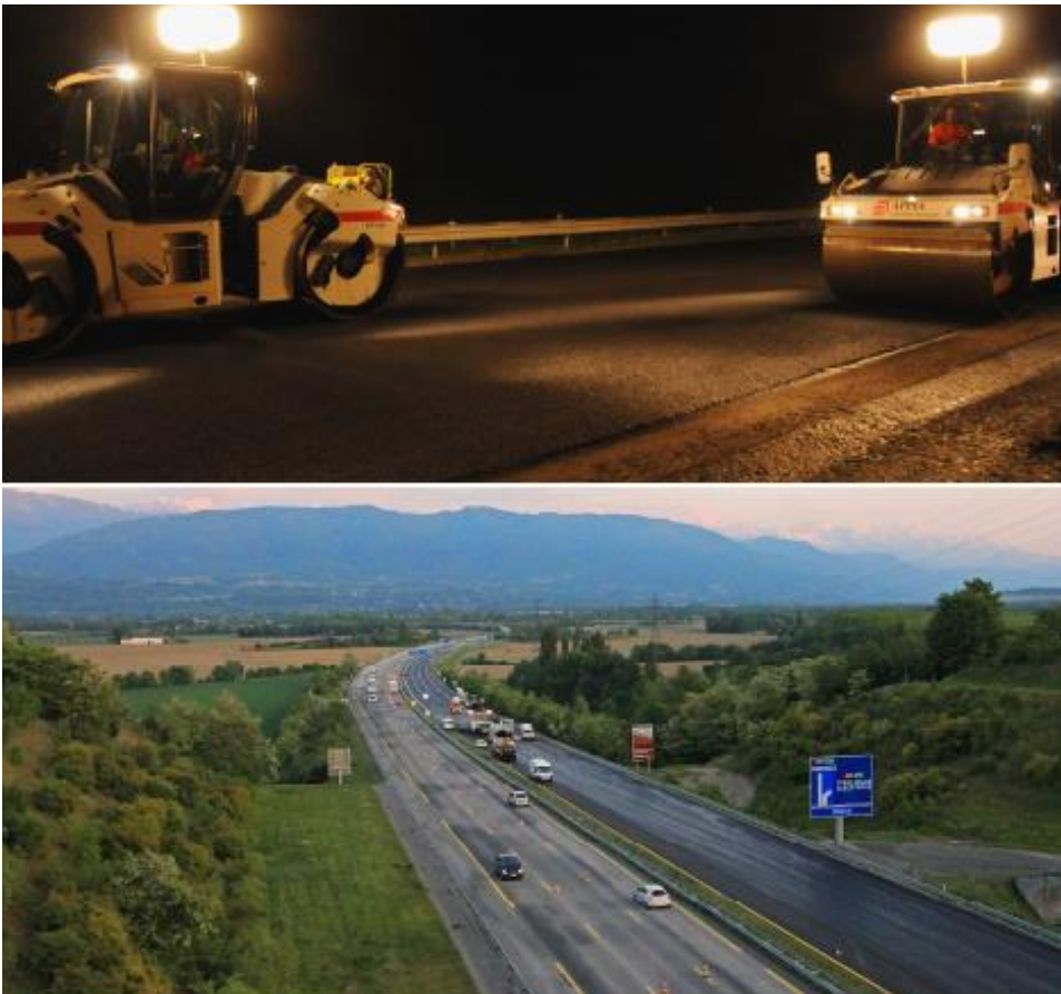
Figure 8: 31,000-ton GB5 ® 0/14 roadwork on the French A41N & A43 toll highway (AREA network) in the Alpine area. SBS-modified binders Biprene ® and Orthoprene ® were both used.
