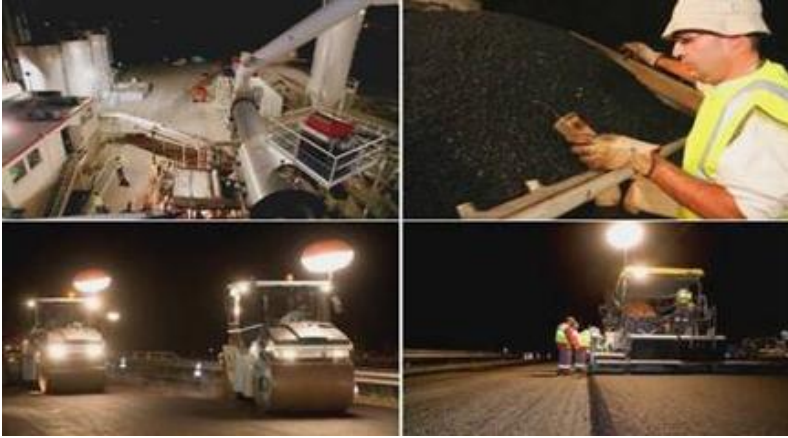
Figure 7: Paving GB5 ® 0/14mm high-performance asphalt with Cemex aggregates, 35/45B binder and 35% RAP (reclaimed asphalt pavement) near Toulouse. In-place density: 97%; modulus E*(15°C-10 Hz): 15,100 MPa.
