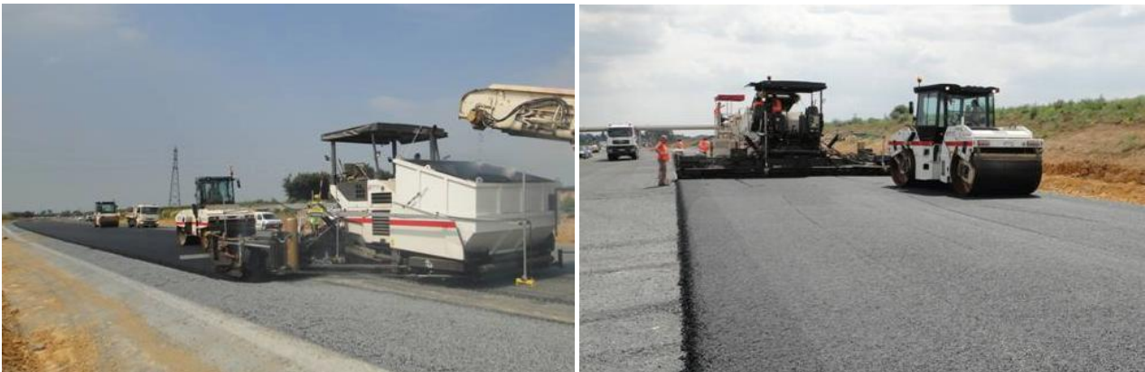
Figure 9: 4,000-ton GB5 ® 0/14 roadwork on the French A13 toll highway (SAPN network, A13-RD613 section) in Normandy. 35/45B bitumen and SBS-modified binder Biprene ® were both used.
