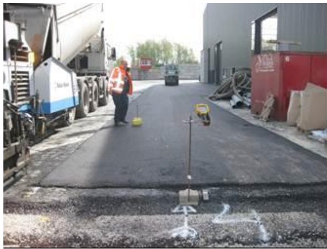
Figure 7: Measuring nuclear density and asphalt temperature by infrared camera and temperature probes in surface layer in track next to factory hall
