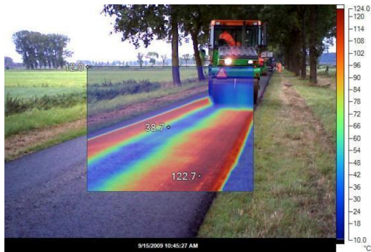
Figure 5; An example of inhomogeneous cooling of the asphalt due to (planned) inconsistent layer thickness
