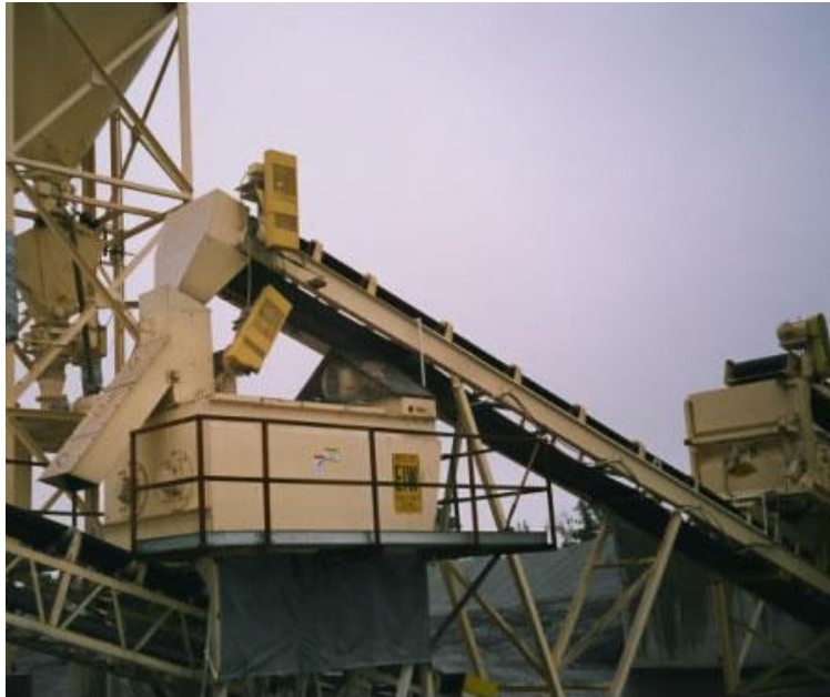
Figure 2: Pugmill used to mix hydrated lime with the wet aggregate in South Carolina (from [11]).
