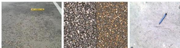
Figure 2. Stripping Phenomenon Evidence in Flexible Pavements
