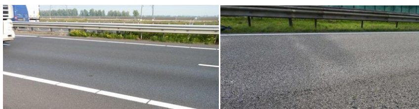
Figure 1: Left: section A15_1995, 15 years in service and hardly damaged. Right: N3_2004, 6 years in service and suffering from severe winter damage.
