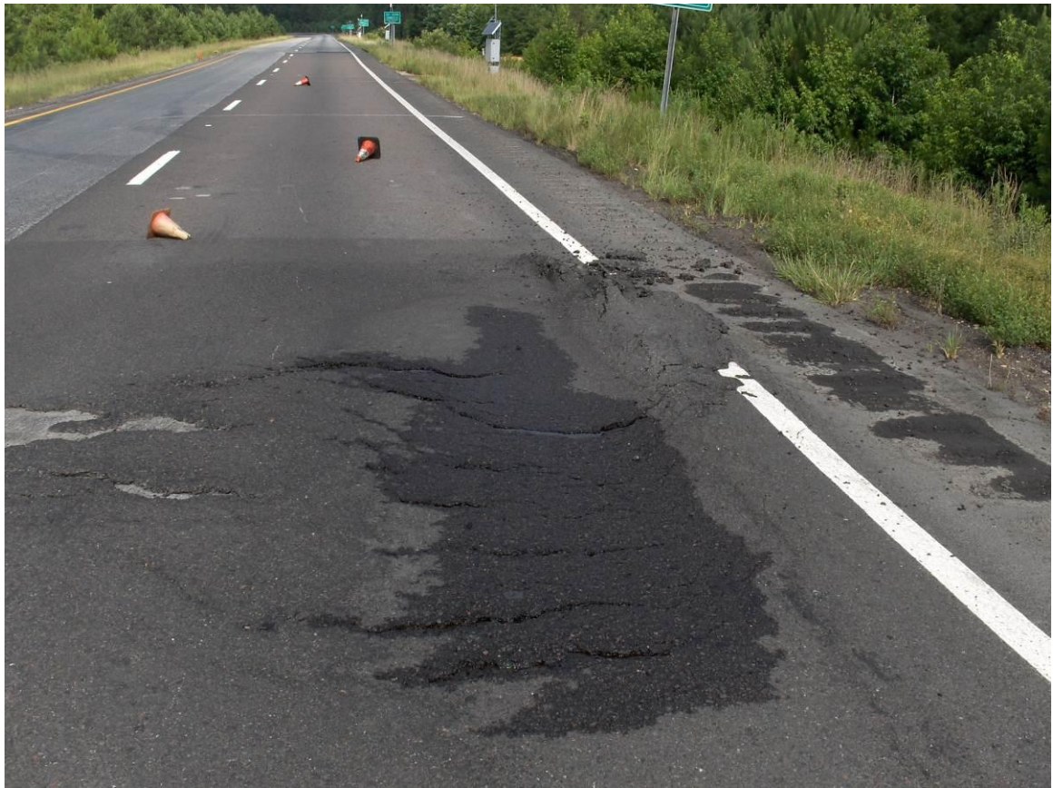
FIGURE 2 : N8 Pavement failure after conventional mill and inlay.
