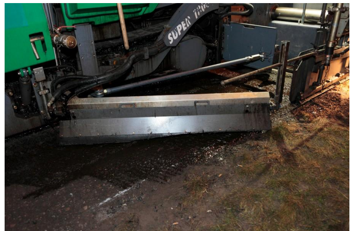
Photo 4: Detail of spray bar
