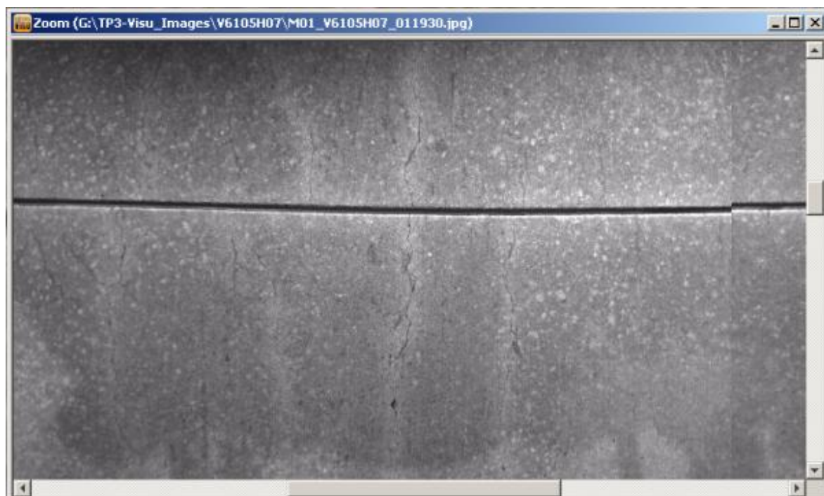
Figure 13: Cracks qualified as caused by alkali-silica reaction (ASR) during detailed analysis using ZEB-Visu
