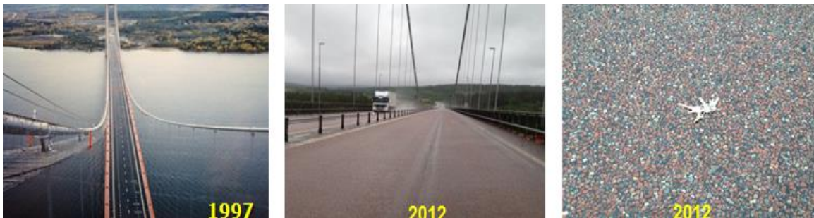
Figure 2: The High Coast Bridge in November 1997 and its pavement surface conditions in June 2012
