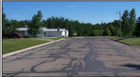
Figure 3. Excessive Crack Filling (Photograph by Dale Decker)
