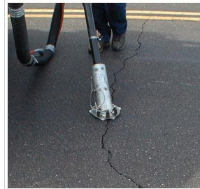
Figure 16: Crack Vacuum (Courtesy Crafcoc)
