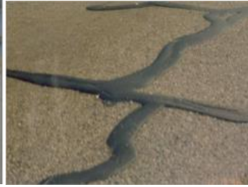
Figure 11 Excessive Overbanding (B)(15)
